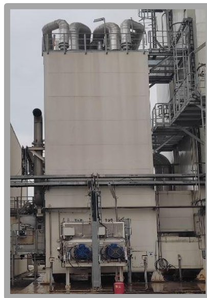
Figure 1.8 Main heat exchanger
