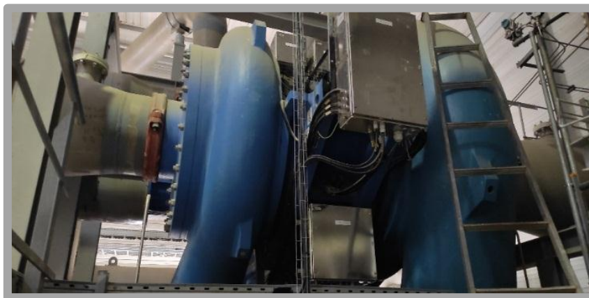
Figure 1.2 Main air compressor
