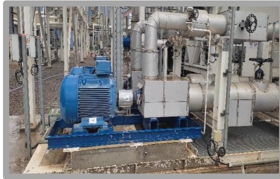
Figure 1.5 chilled water pump
