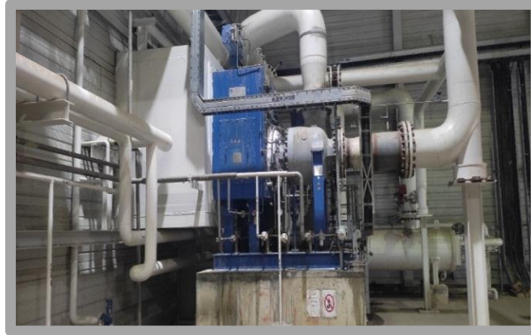
Figure 1.7 Expansion turbine and booster
