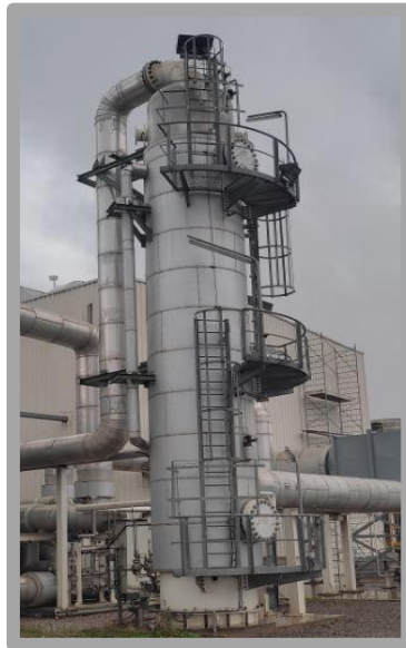
Figure 1.3 process air cooler
