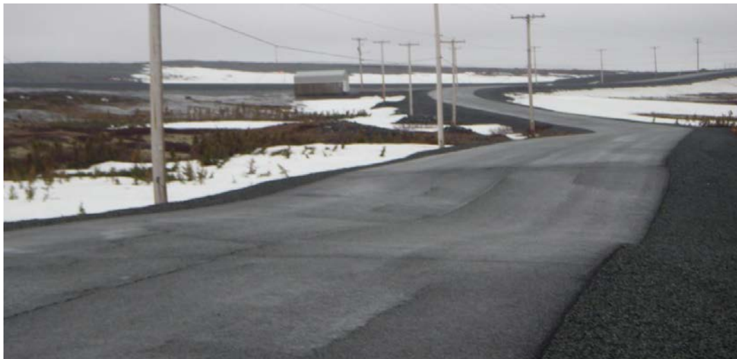
Fig.18. Tassement de route
