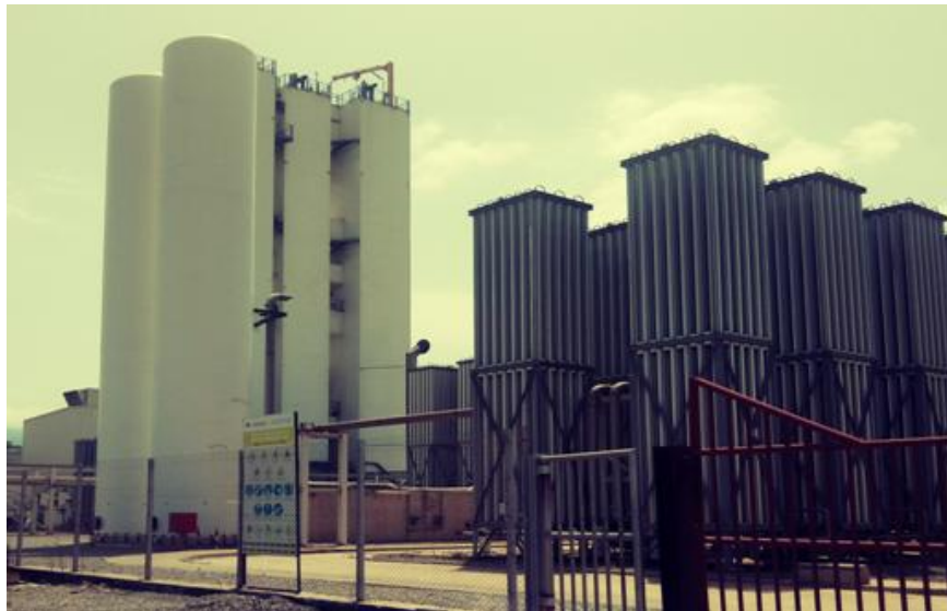
Figure I.5. Air Separation Unit.
