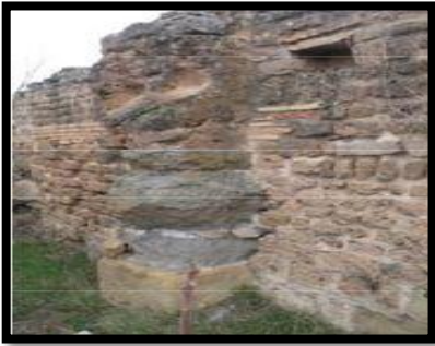
Figure n° III .18 : Les grands thermes, dégradation due aux restaurations abusives
