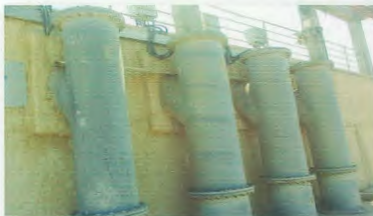
Figure 6: La station de relevage
